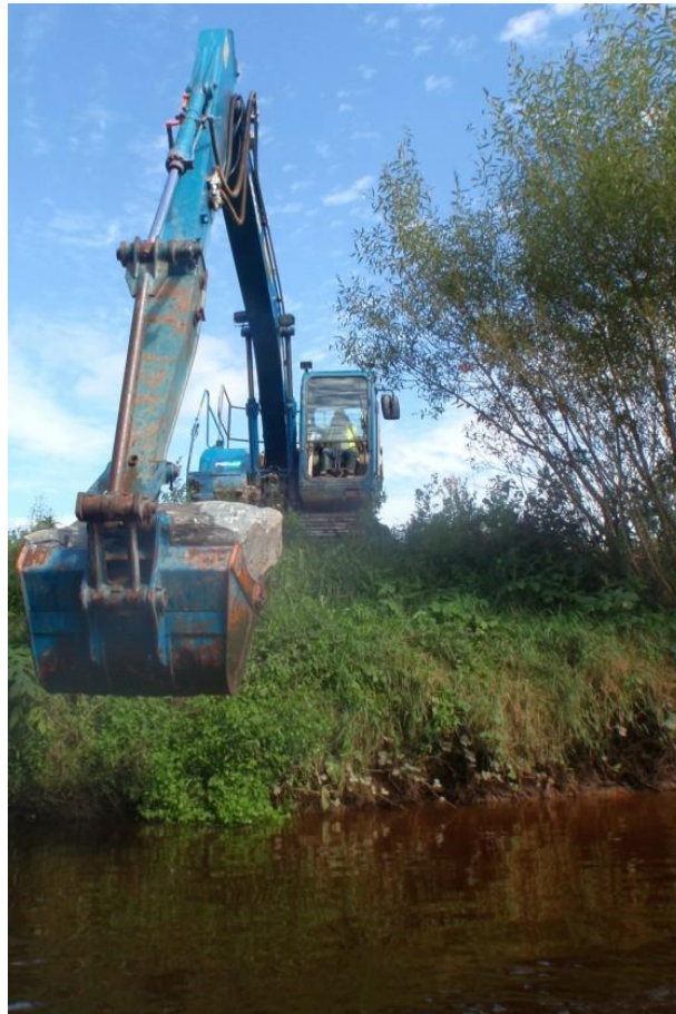
Skilled OPW staff use hydraulic excavators to precisely place rock (Image: Glen Wightman)
