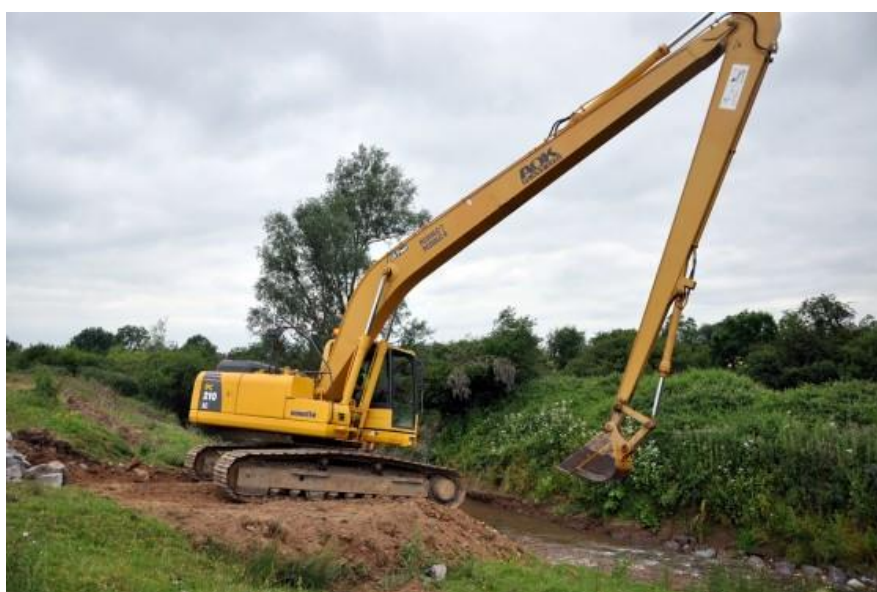
Skilled long-reach excavator driver works from the bank (Image: Ruairí Ó Conchúir)
