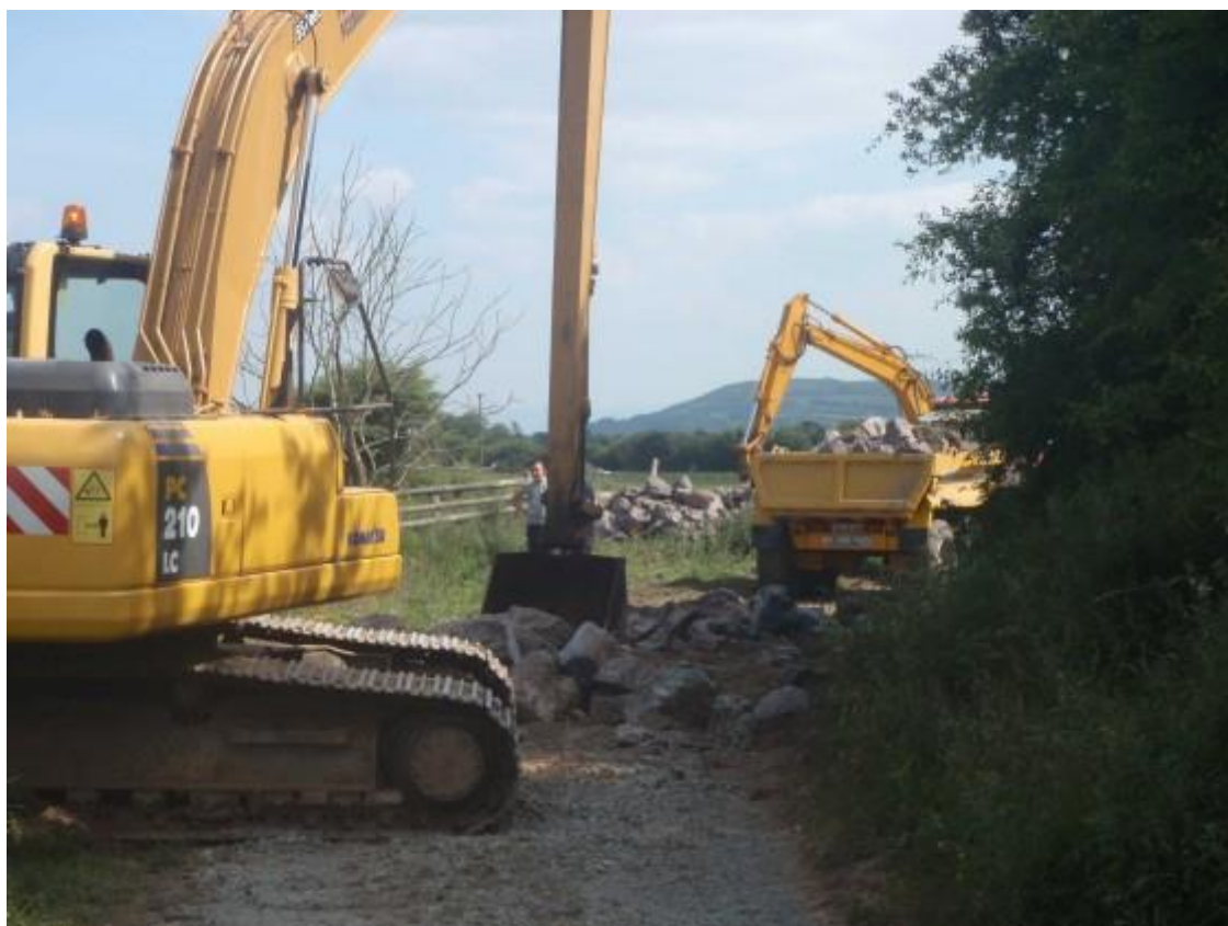
*Large quantities of rock are used to complete instream works (Image: Glen Wightman)
