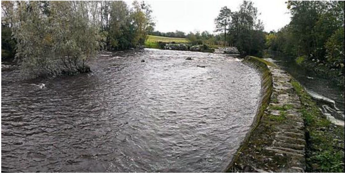
Panoramic view of the completed work at Ballyclogh weir (Image: Martin O' Grady)
